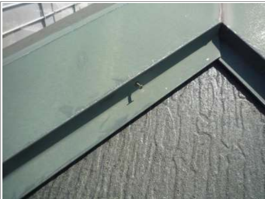
棟鉄板補修施工前
